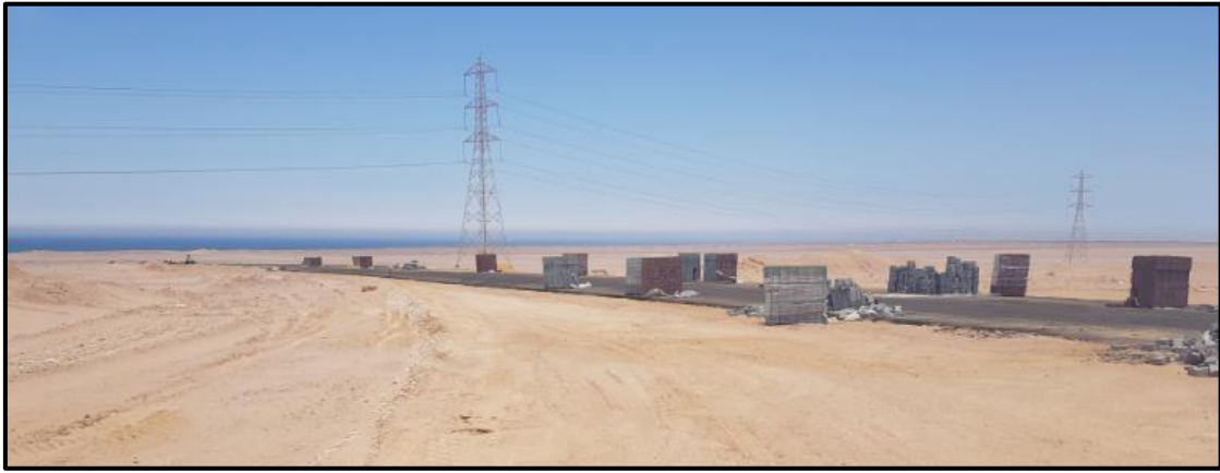
Figure 17: Road Currently under Construction that Links a Wind Farm Site to Hurghada-Ismailia Road
